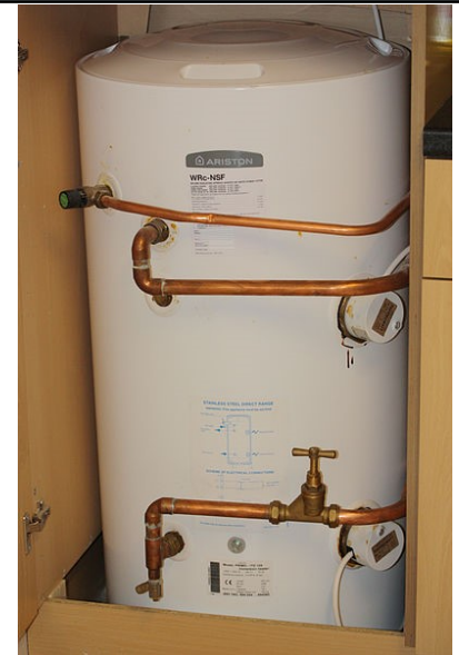
Hot water storage tank in a UK property. Workman (2010)
